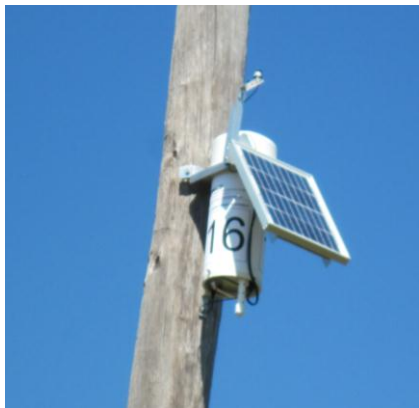
Fig. 3: NEO Secondary DAS installation.
