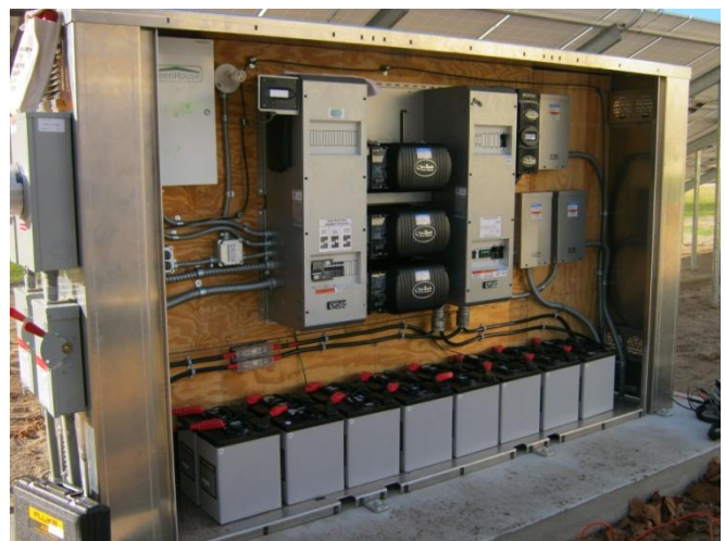
Fig. 2, Metal enclosure with balance of system components.
