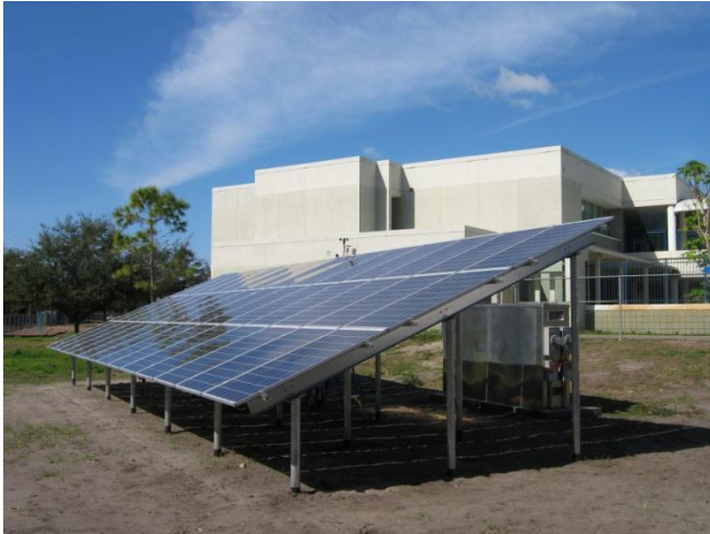
Fig. 1. PV array at Fairmount Park school.
