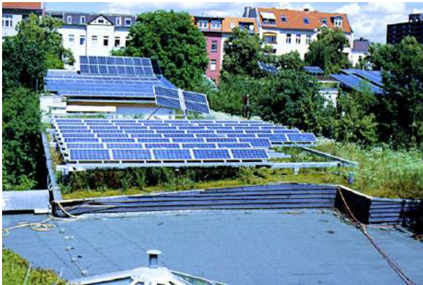
Fig. 2: The GRIPV system with intensive green roof and monocrystalline PV in Kohler et al., 2002.
