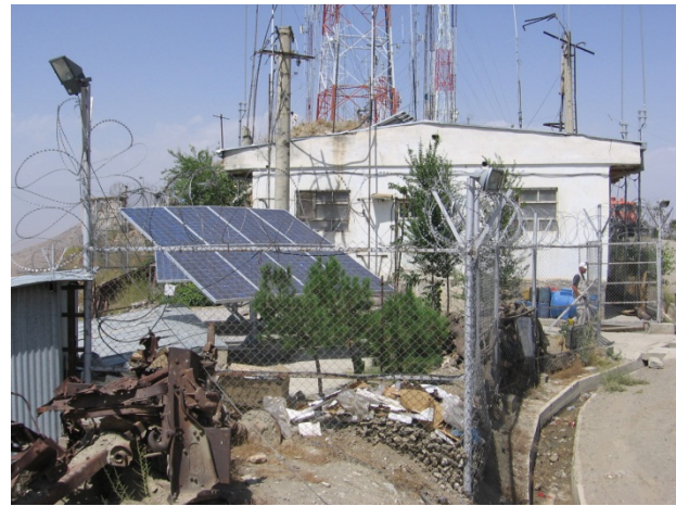
Fig. 5: Typical Radio Site With Solar Power
