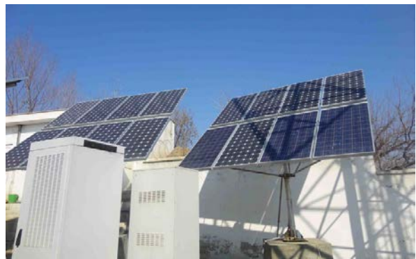
Fig. 8. Example PV Installation Afghanistan Cell Site
