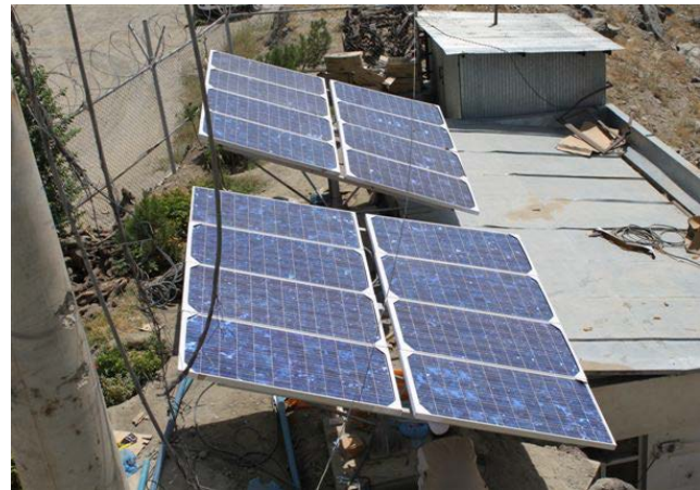
Fig 3. Radio Site Solar Power
