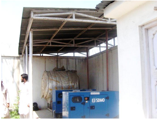
Fig 2. Point of Use Generator at Radio Site
