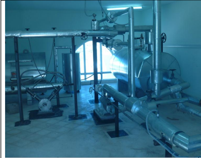
Fig. 3: Power plant room
