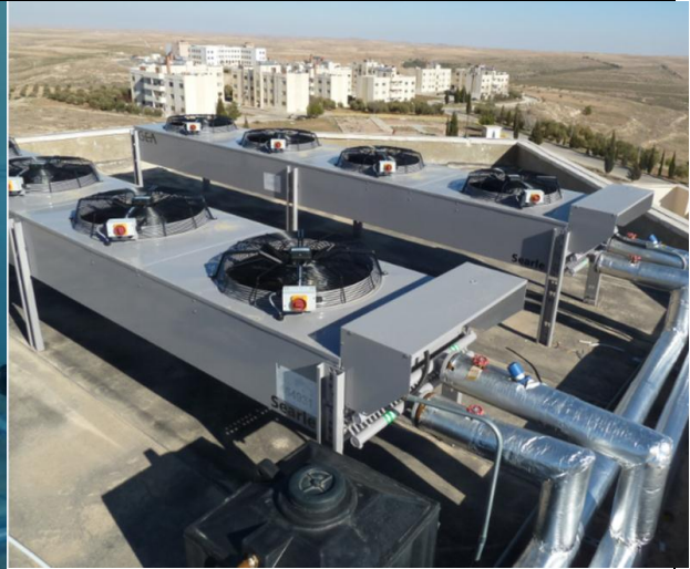
Fig. 4: Dry cooler for the Chiller
