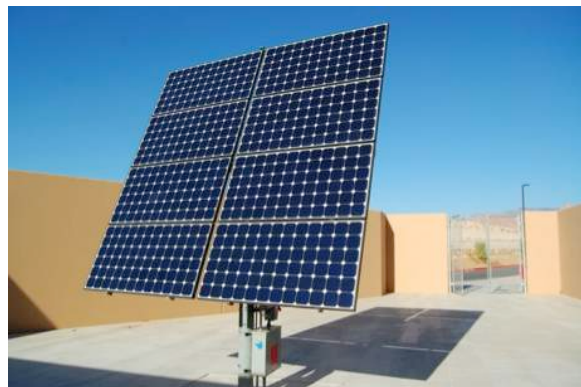
Fig. 9: Solar PV installation at West Career & Technical Academy.
