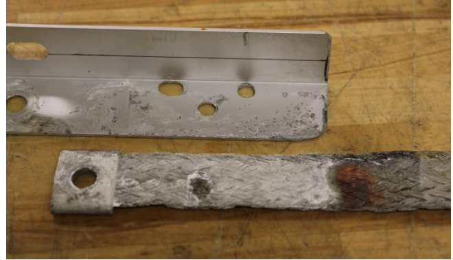
Fig. 6: Corrosion at unprotected edge of aluminum angle
