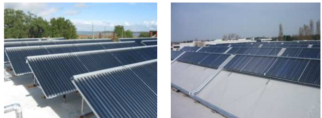
417 m 2 Parris Island (USA 2011) cooling 550 m 2 Kral (Austria 2011) cooling
