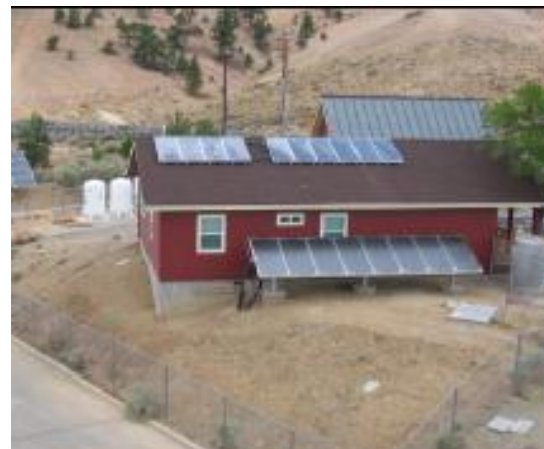
Fig. 4: Solar Array 1 (rack mounted), Solar Array 2 (roof mounted); Workshop solar-roof air heater in upper right background.
