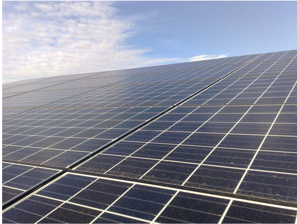
Solar panels atop EBU2 building on the UCSD campus.
