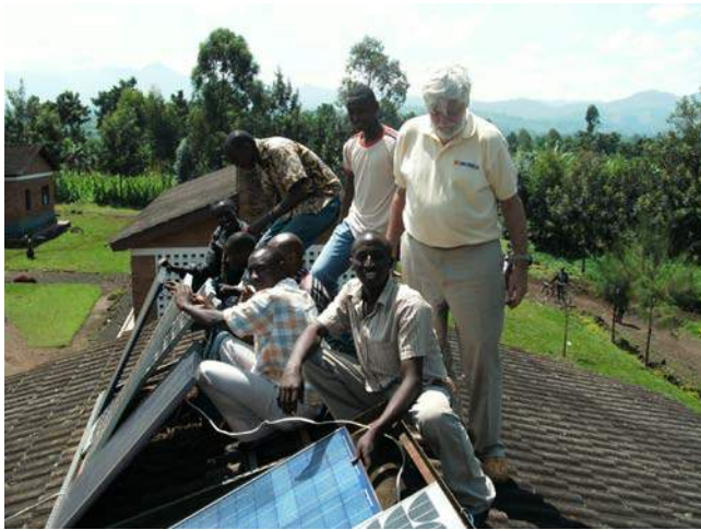
Fig 8 Richard Komp helping the Radiant Horizon group find the problem (a broken wire) on a non-functional PV array on a health clinic in Rwanda.
