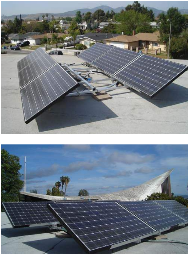
Figure 5: Two views of a 1.2 kW (peak DC) JXC SunTrack Carousel mounted on a church rooftop in San Diego CA.
