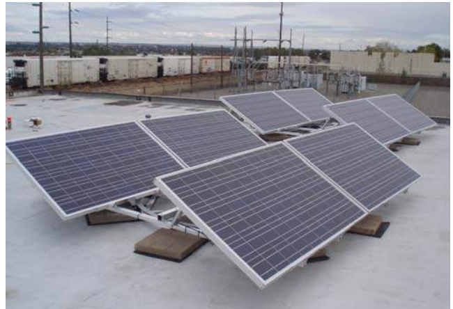
Figure 3: The two JXC SunTrack Carousels shown here were installed in Eastern WA in October of 2007.
