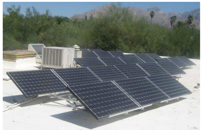
Figure 4: Four JXC SunTrack Carousels on rooftop in Tucson AZ (4.68 kW). Six Sanyo modules are mounted on each carousel in 2 rows with 3 modules per row.
